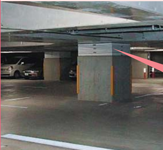
Seismic base isolation structure of the new Kure Plant building, as seen from the basement parking lot
