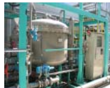
New circulating water system
