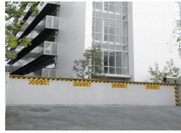
Tide protection gate
