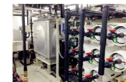
Waste water recycling equipment
